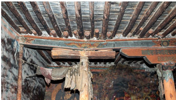
Figure 456: The broken beam with additional support before restoration.
