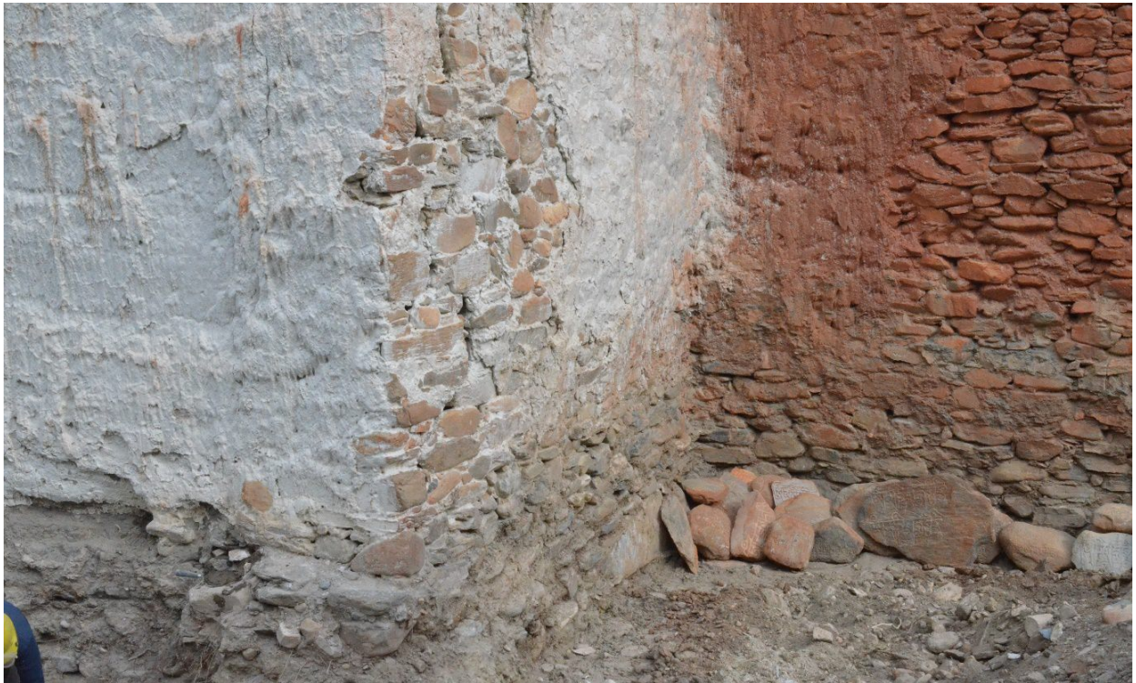
Figure 190: View of the northwest corner with the wall cracked and bulging.
