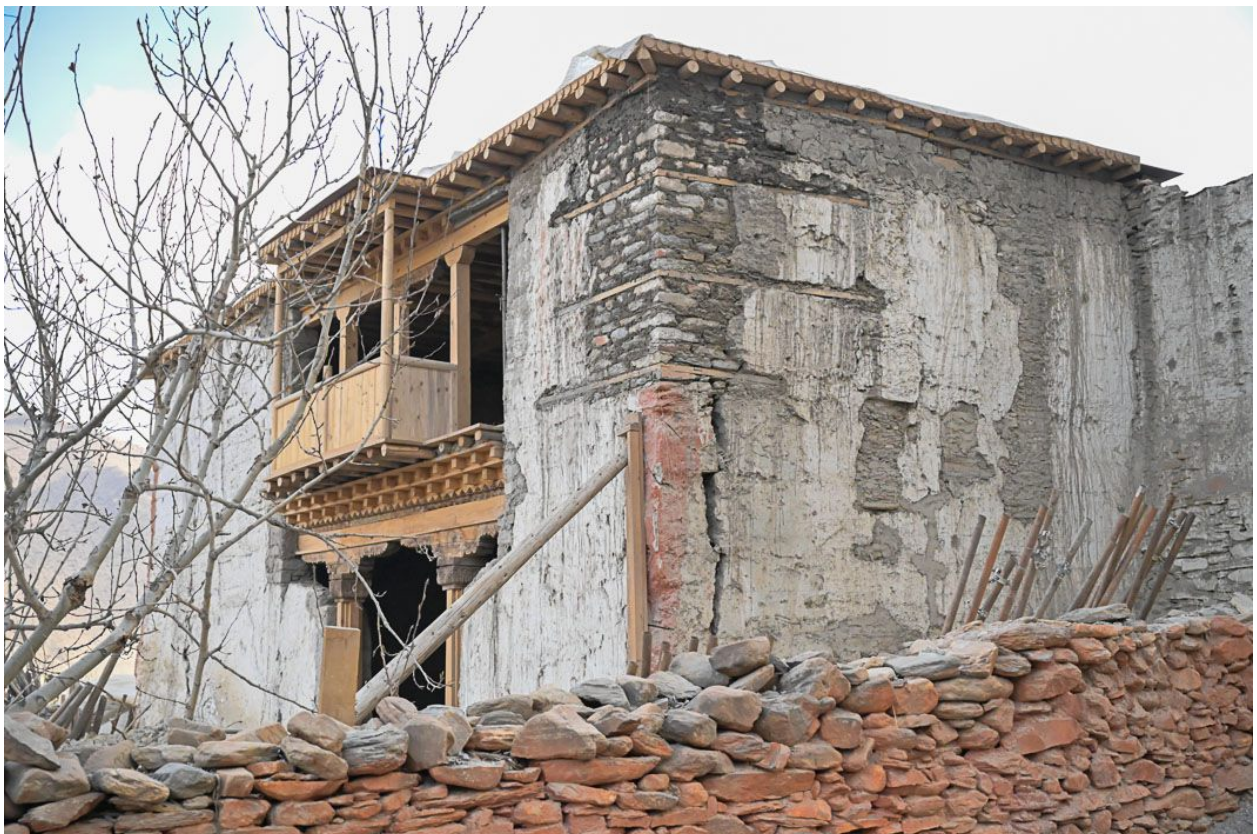
Figure 128: The northeast corner after reconstruction, the crack still visible on the lower floor.
