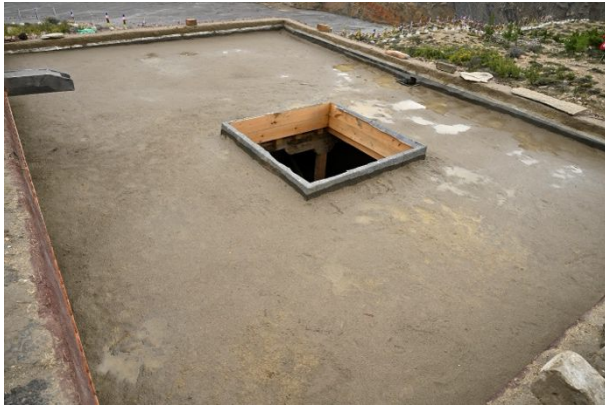
Figure 336: Part of the South Wing with two mud layers after two days of heavy rain. There was no leakage but the water did not run off completely either.
