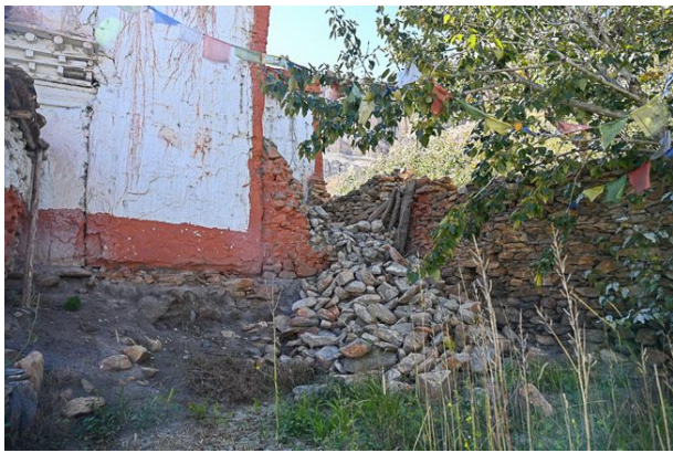
Figure 41: Stones from collapsed wall in front of the temple.
