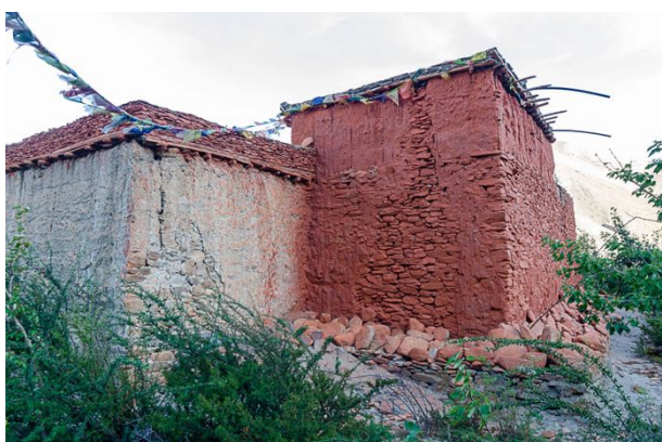
Figure 441: The northwestern corner before restoration.
