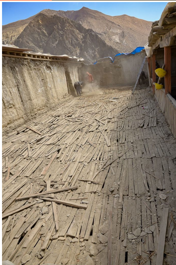
Figure 246: The wooden splits covering the ceiling of the lower level after removal of all the mud.
