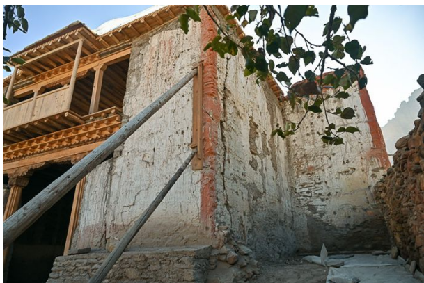
Figure 121: The severe crack at the northeast corner of the Entry Hall in October 2023.
